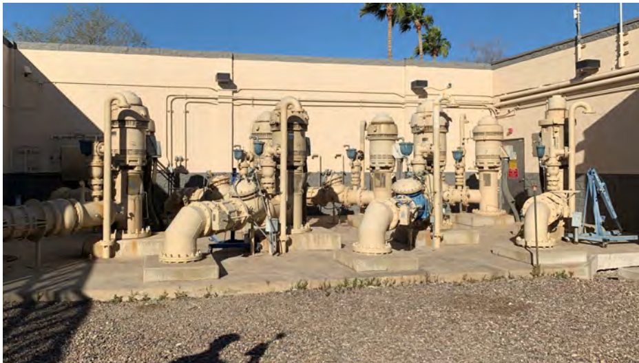
Figure 1: Booster Pumps X2
