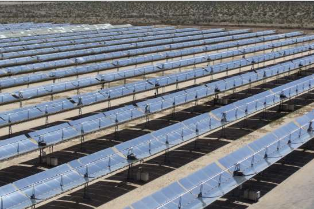
View of the Solar Collector Assemblies
