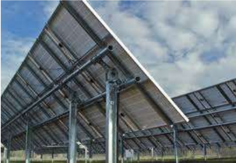
Example of PV Solar Field showing underneath side of solar panels
