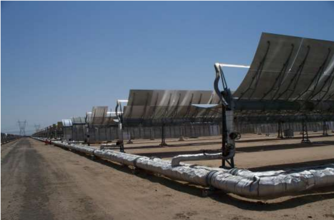
Existing field showing mirrors, piping, and heat collector elements
