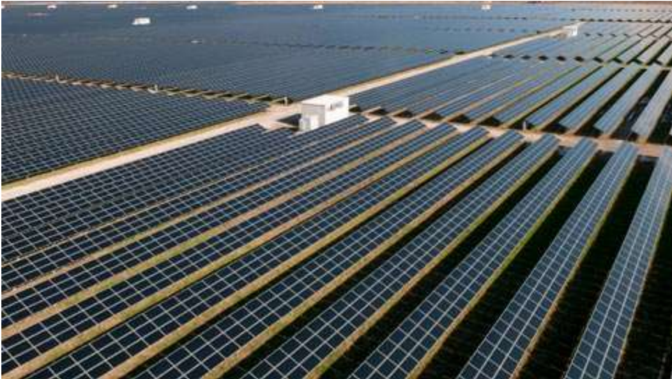
Example of PV Solar Field with transformers and inverters shown
