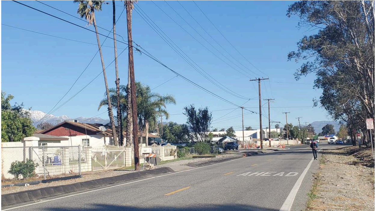
Figure 6: Deficient Pedestrian Infrastructure on NB Alder Ave
