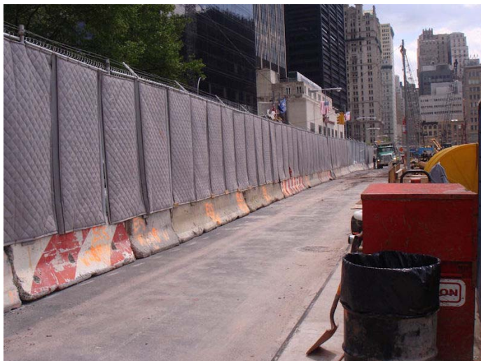
K-Rail Temporary Fence & Acoustic Material
