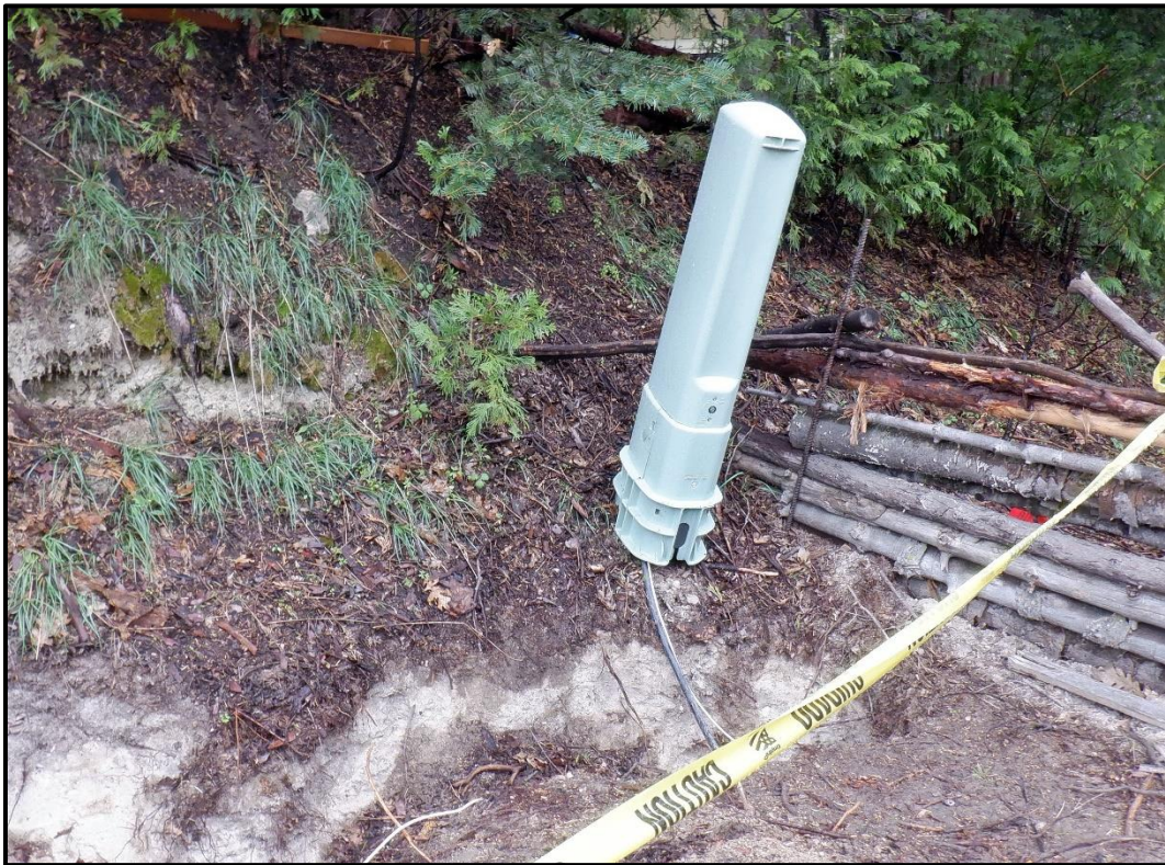
Figure 10. Modern Utility Box and Exposed Wires within Property.
