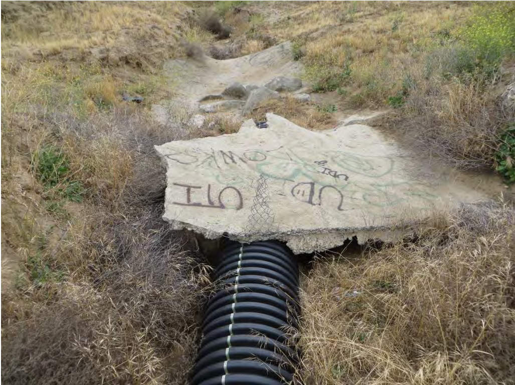
Photograph 4: Facing east along Drainage A at an exposed culvert and concrete reinforcement within the drainage.
