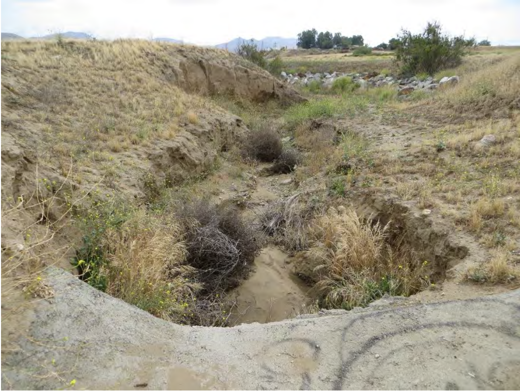
Photograph 5: Facing east along Drainage A, with a riprap-reinforced detention basin in the background.
