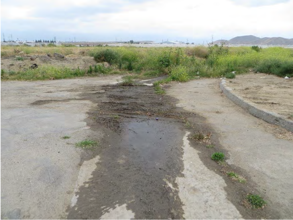
Photograph 1: Facing east from the corner of Del Mesa Drive and Halbrook Lane into Drainage A, which is fed by water runoff from the adjacent neighborhood and surface streets.
