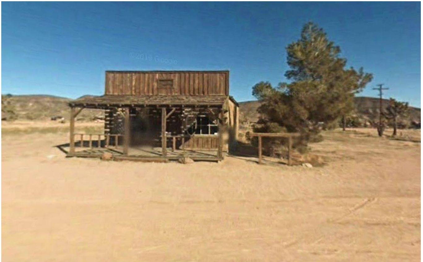
Photograph 1: Looking north from Mane Street at the front of the existing vacant building.
