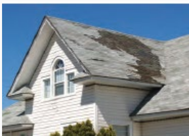
Roof cladding damage.
