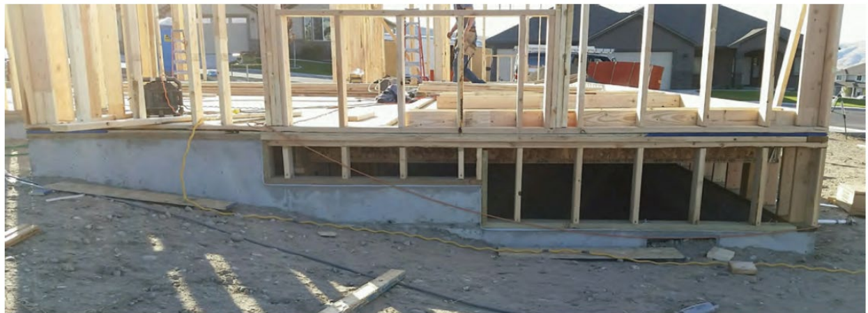
Cripple wall along exterior of house – unsheathed.
