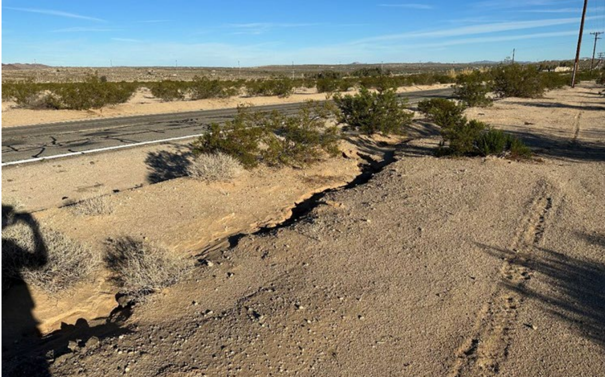
Photograph 11. Surface flow along western perimeter of Parcel 061213101, facing northwest.
