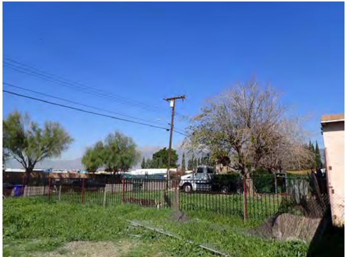
16) View of the pole-mounted transformer on Calabash Ave.
