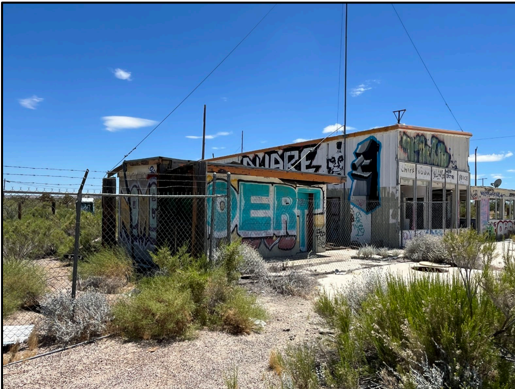
Plate 3.2–4: North façade of ancillary storage structure with north and east façade of the former gas and service station building in background, facing south/southwest.
