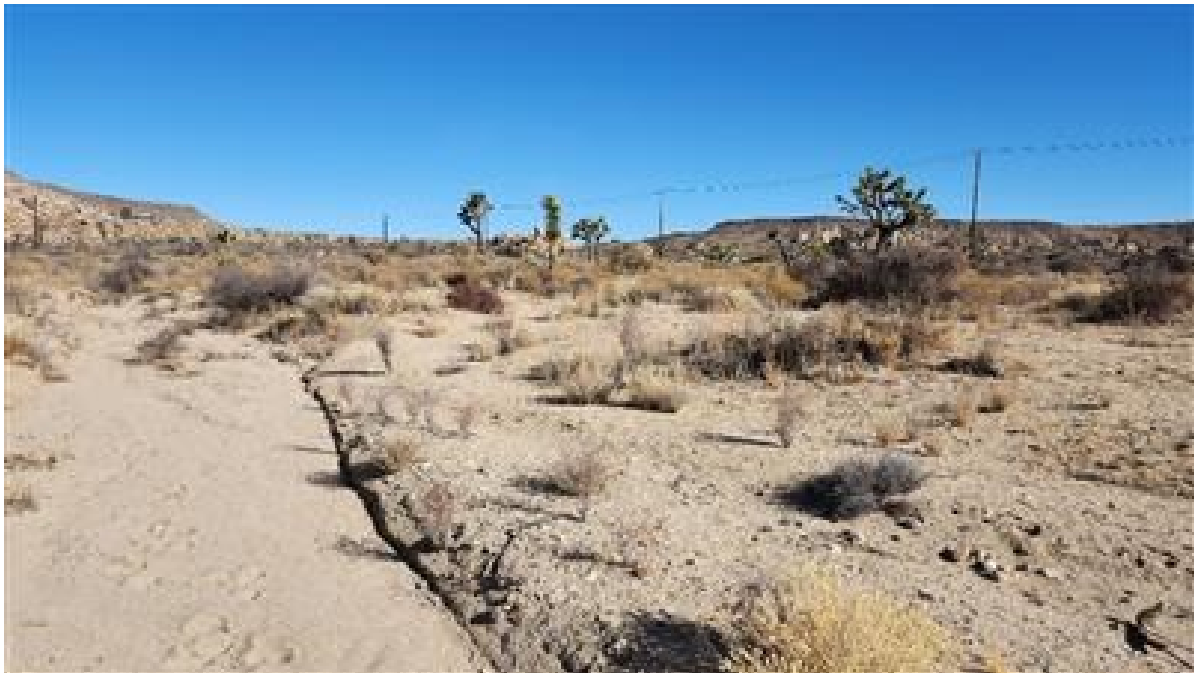
Photo 6. View from within Drainage #1 approximately 75 feet southeast of photo #4 and #5, facing northwest.
