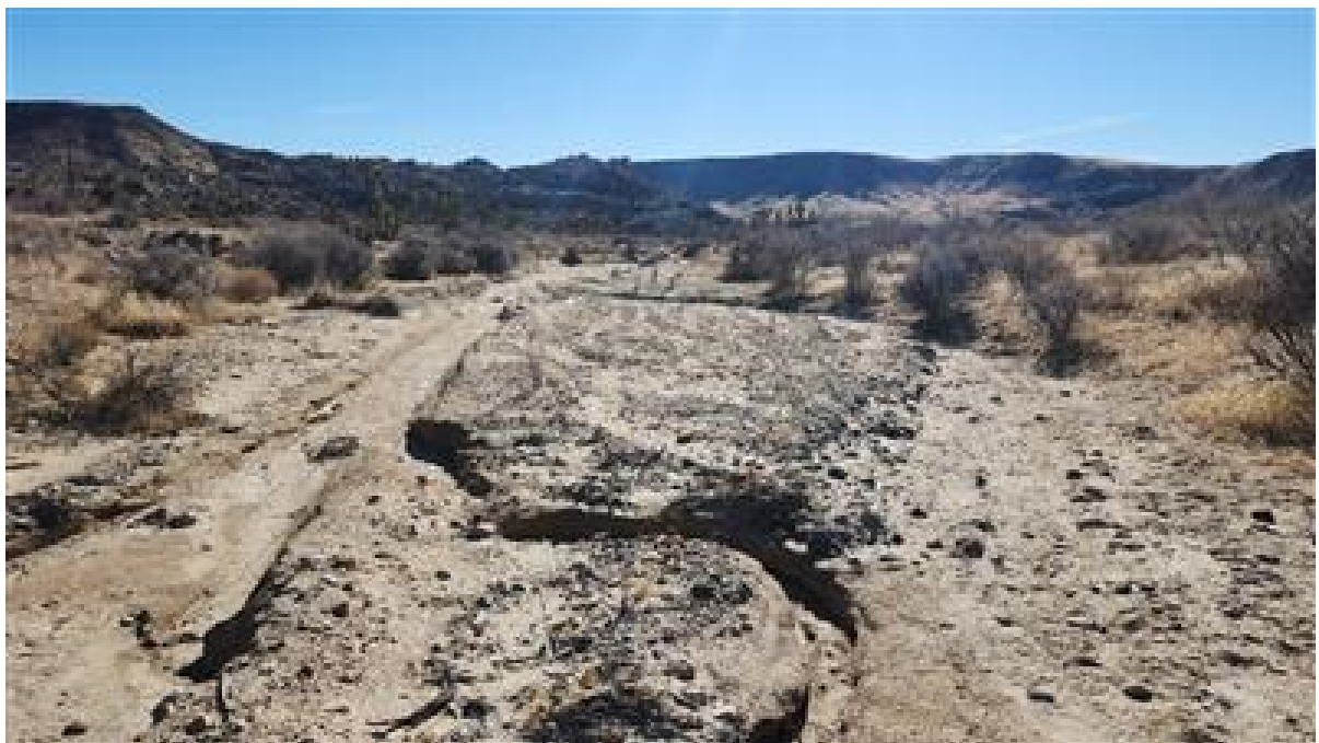
Photo 2. View from within Drainage #1 approximately 150 feet southeast of photo #1, facing southeast.
