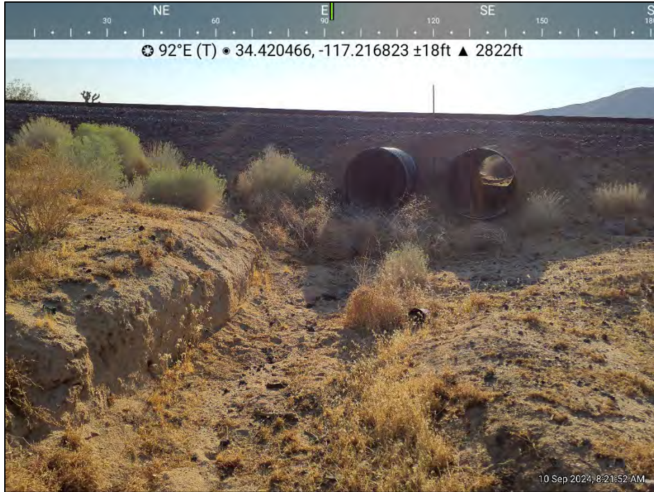
Photo 5. Feature 1 Enters the Northeast Portion of the Study Area Through Two Side-by-Side Culverts Located Underneath a BNSF Railroad Track.
